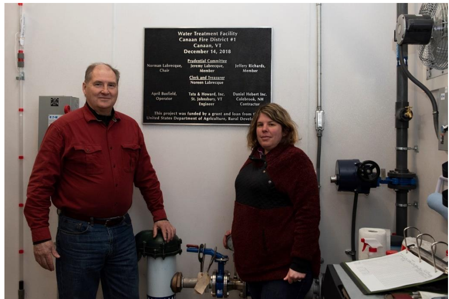
April Busfield (right) and Gary Leach at Canaan Fire District #1. Credit: Vermont Rural Water Association
